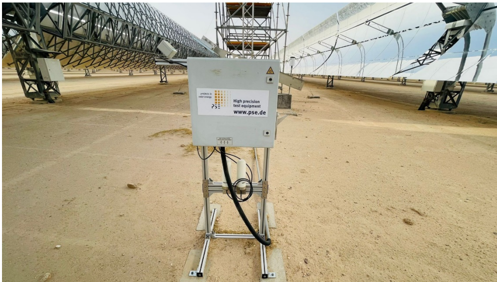
AVUS-Sensor: Soiling measurement at the Shagaya parabolic trough power plant built by the TSK group and owned by KISR (Kuwait Institute for Scientific Research). © TSK-Flagsol
